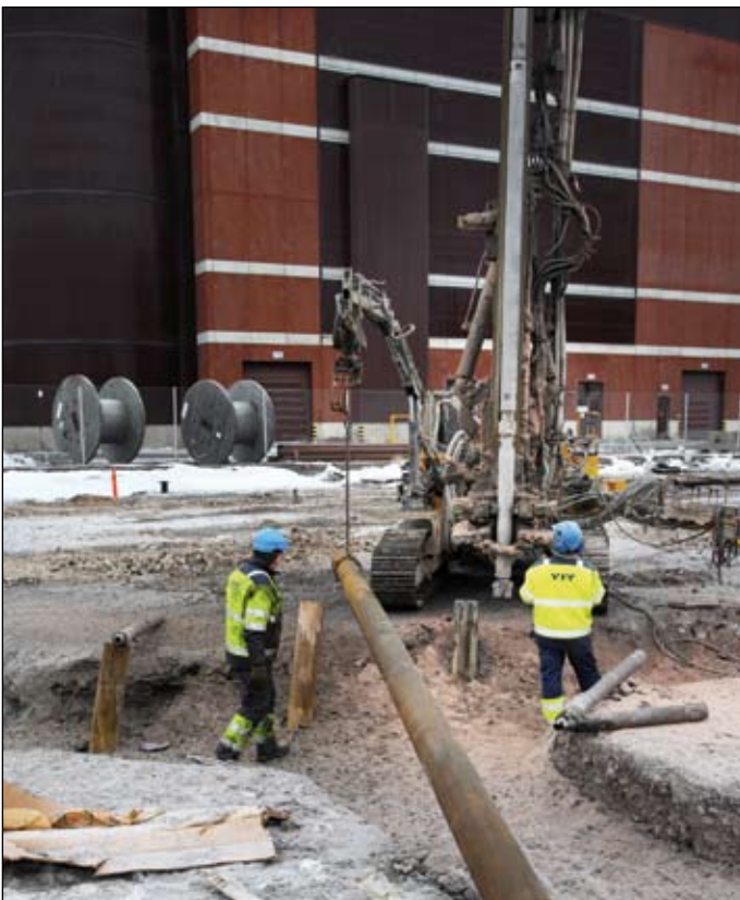
The pile casing, a drilling pipe during installation, and part of the load-bearing pile structure.
