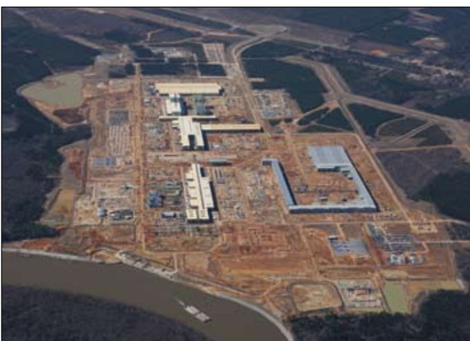
Since 2007 ThyssenKrupp Steel USA and ThyssenKrupp Stainless USA have been working together for the erection of the new plant for steel and stainless steel flat products in Alabama.
